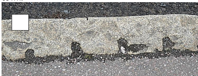
Pavement edge in Fore Street showing the drill holes where the granite was split – can you find it?
